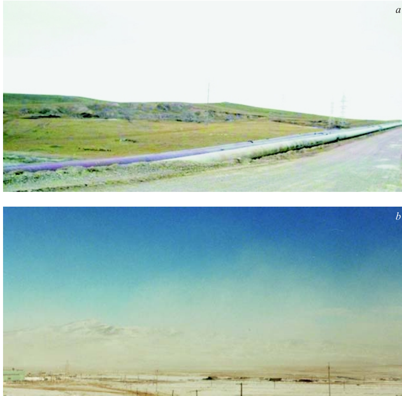
Fig. 2. The double pipe of tail's pulp to the storage of Slag-heap tail (a); white sand or dust of the storage of Slag-heap tail (b)
